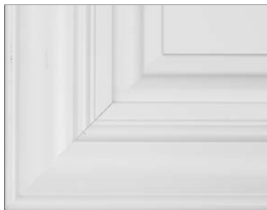
Example of front joint separation
