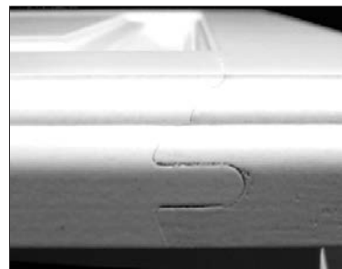
Example of end joint separation
