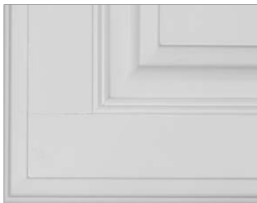
Example of front joint separation
