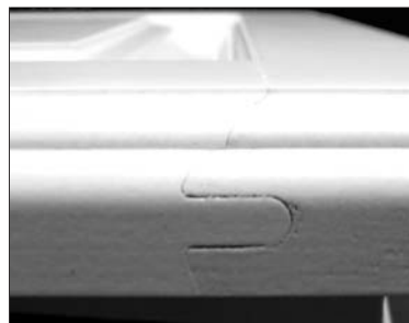
Example of end joint separation
