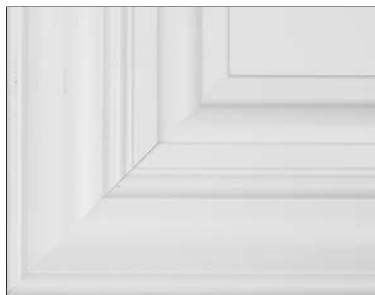
Example of front joint separation
