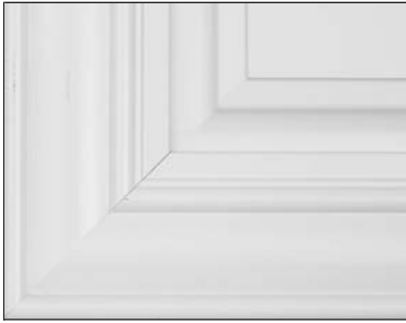
Example of front joint separation
